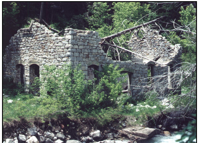
Fig. 2. The Columbus Power Plant as seen in June 1996. The roof is completely gone and a large tree has fallen across the side walls, taking down many of the stones. The stone wall along the creek has been washed away, but the tail race conduit for the east generator still extends out into the stream.
