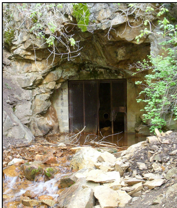
Fig. 2. The portal of the Mutual Metal tunnel has a steady stream of water flowing from it. The torn metal mesh barrier is barely visible in this photograph.
