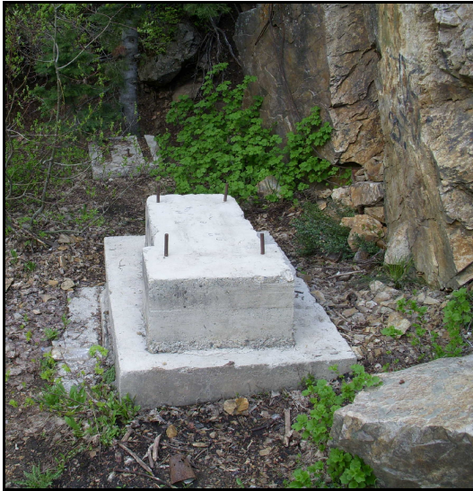
Fig. 3. Concrete foundations for the air compressor and its electric motor are on the south side of the tunnel's portal.
