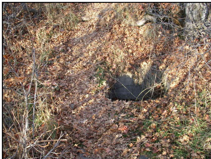
Fig. 3. An Overflow Manhole, once closed by a wooden cover, is at the trail side, posing a threat to the unwary hiker.
