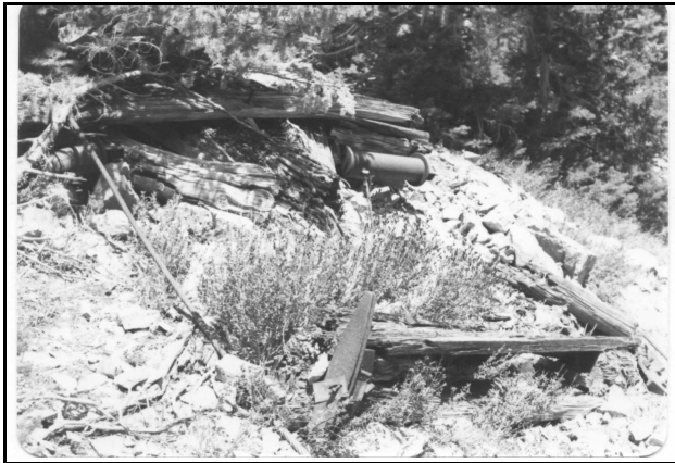
Fig. 4. Remains of a tramway tower that has fallen down hill. The upper cross arm with its carrier casting is in the foreground. The lower cross arm with its rollers is in the background, and the heavy cable crosses from top left to bottom center.
